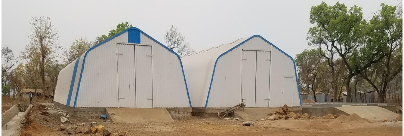
Fig 31:- Three completed platforms and surrounding drainage ditch construction Nguenyiel Refugee camp, Gambella
