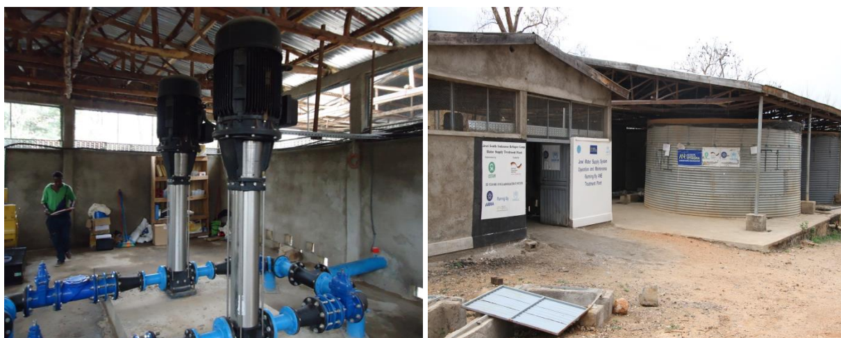
Fig 2:- Treatment system in Jewi
