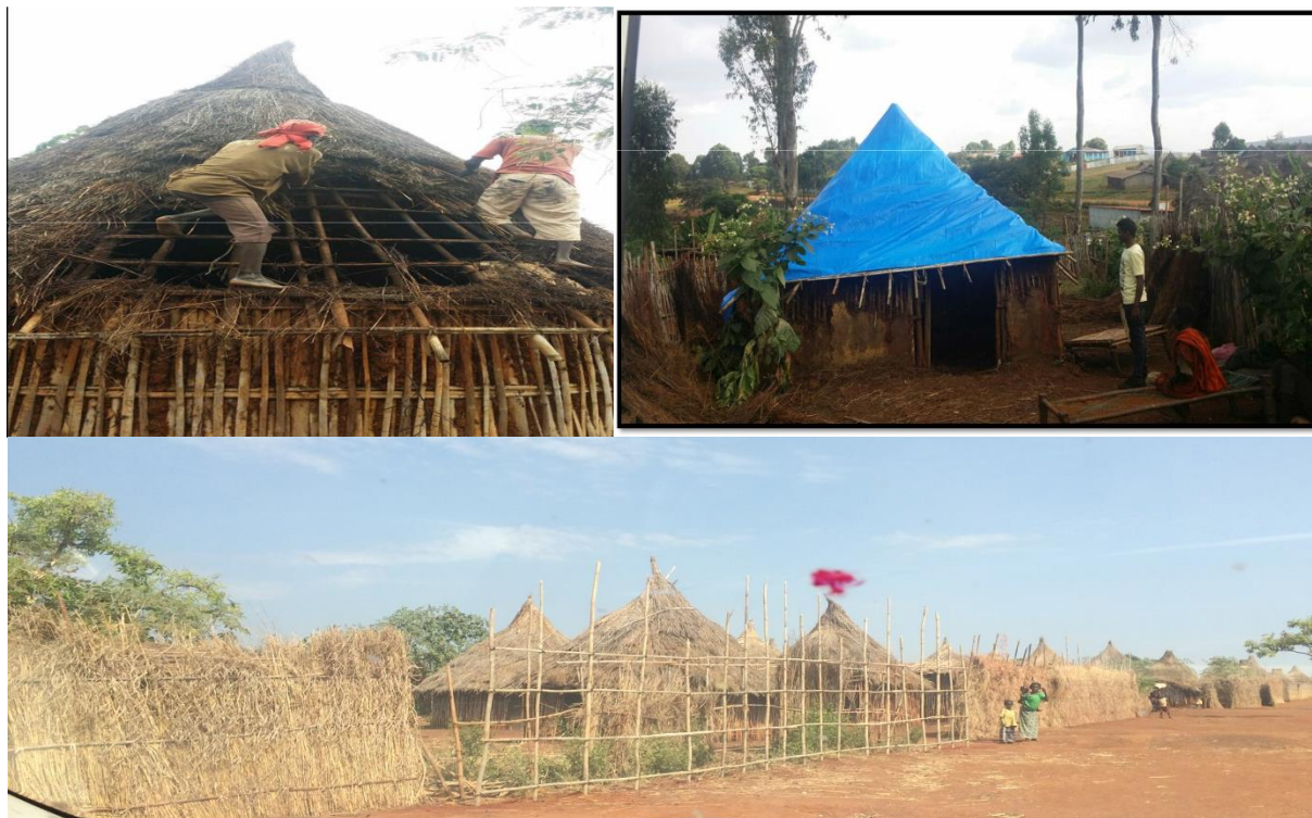
Fig21:-Transitional shelter Maintenance at Bambasi (Assosa)
