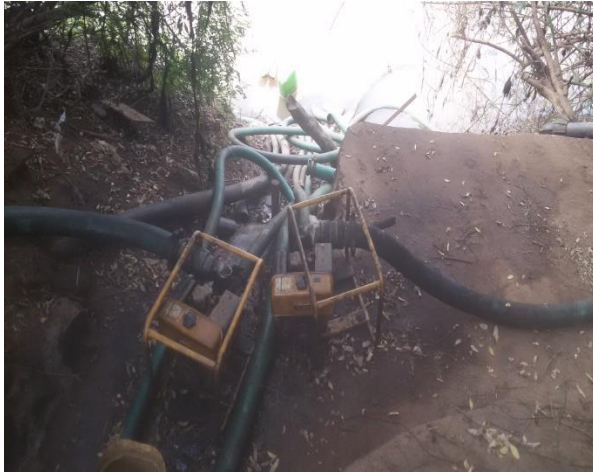
Fig 3:- Intake System In Jewi
