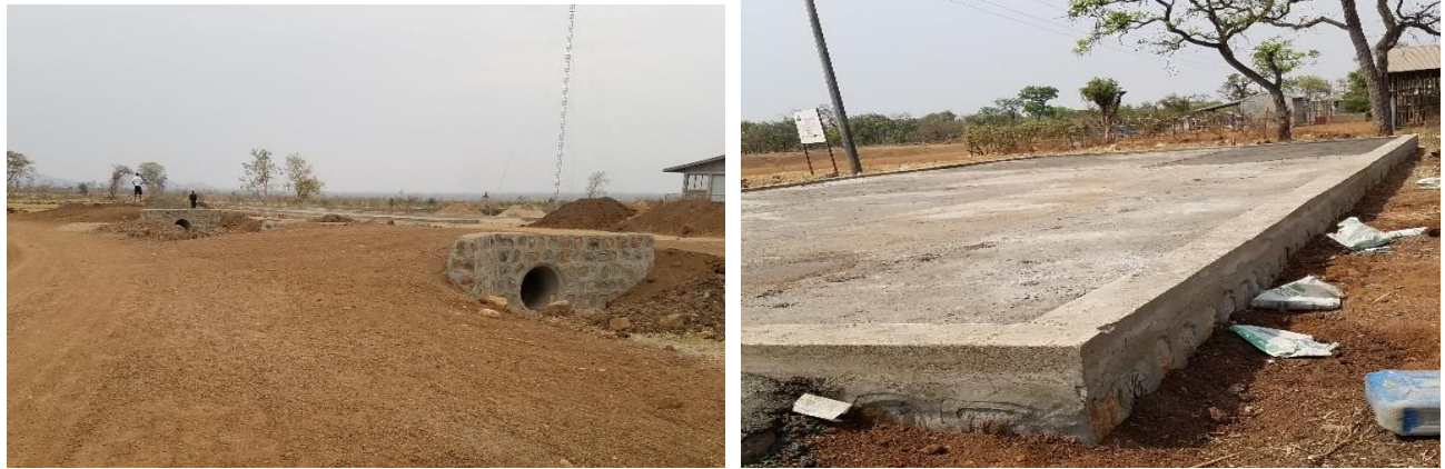
Fig 34 & 35:- Biometric center compound improvement work at (Zone D) Tierkidi Refugee camp (Left) & Completed platform at Akula Camp, Gambella
